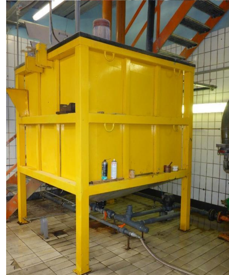
wastewater pre-treatment at atelier CFF, Yverdon-les-Bains
