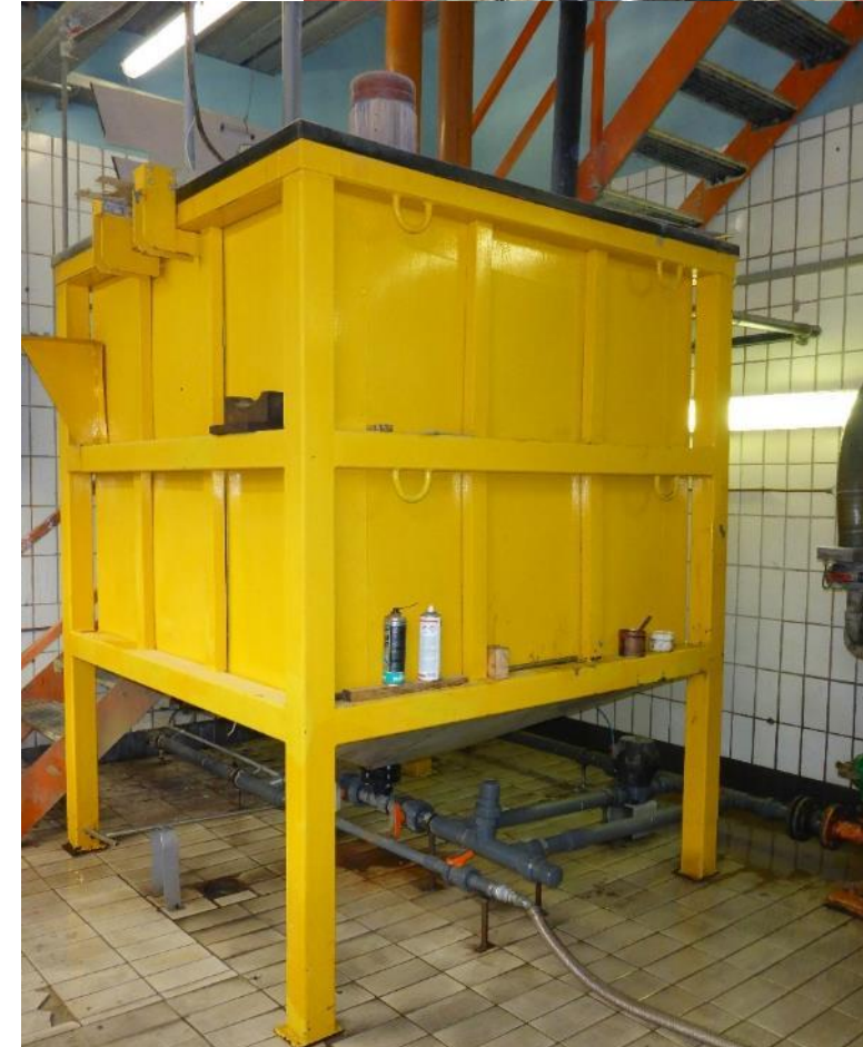
wastewater pre-treatment at atelier CFF, Yverdon-les-Bains
